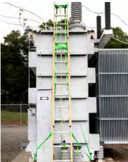
BLT attached to transformer (low mount).
