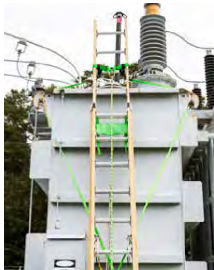
BLT attached behind lifting ears of transformer.
